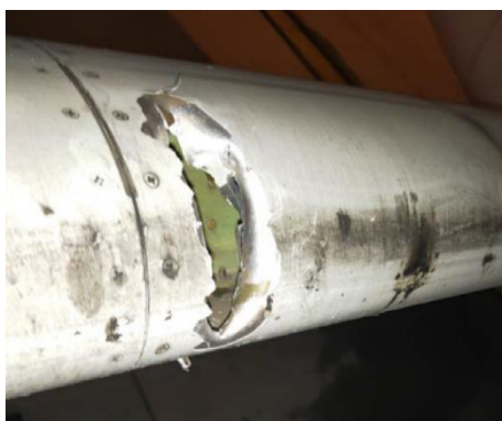
Figure 3-8 Impact Damage on Slat induced by Maintenance Tool
