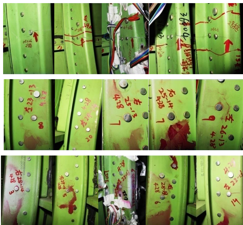
Figure 6-10 WFD of the fuselage frame
