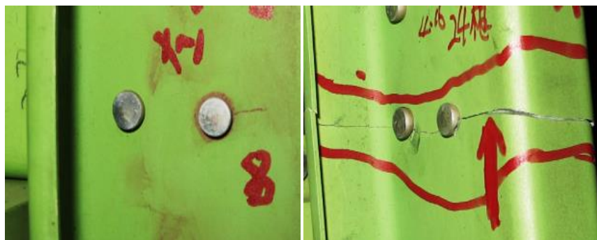
Figure 4-17 Photo of the damaged frames
